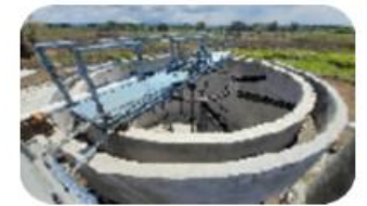
Tertiary treatment (Clarification)
