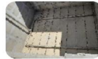
Secondary treatment (Aeration)
