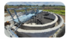
Tertiary treatment (Clarification)
