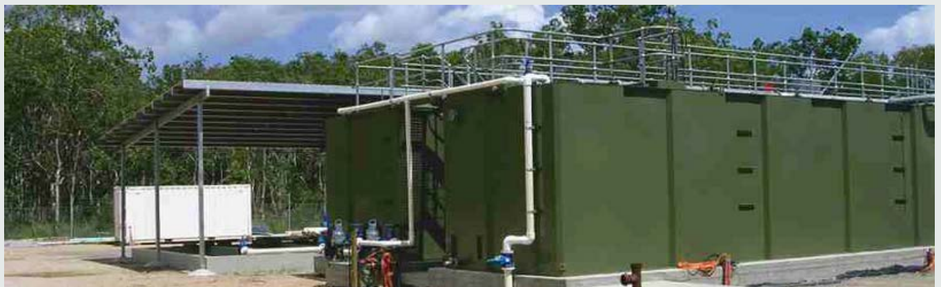
Effluent Recycle Plant
